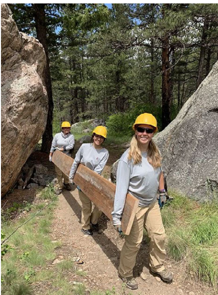
Rocky Mountain Conservancy High School trail crew carrying up lumber for the Young Gulch Trail bridge
